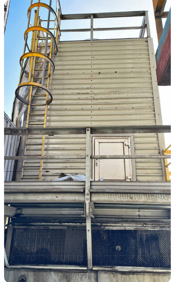
1I RH Cooling Tower
