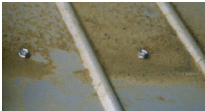
Mould growth on pre-finished steel cladding.
